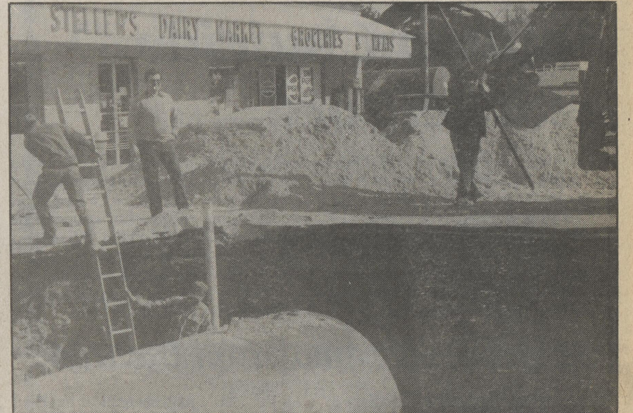
Dave Steller looks on as workmen pipe in one of the new gas storage tanks that was installed Monday morning. The work is expected to take 4-5 weeks. When completed the pumps will have a 45' canopy over them. Photo by Don Mitchell.
